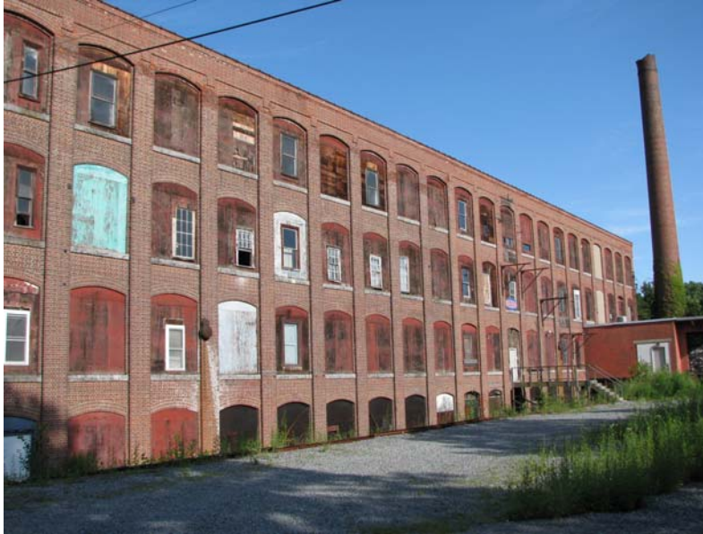
This view of the former Waterhead Mills, now used in part as Romahlo's gym, is looking southeast from the Wamesit Canal. Photo by Gray Fitzsimons.
